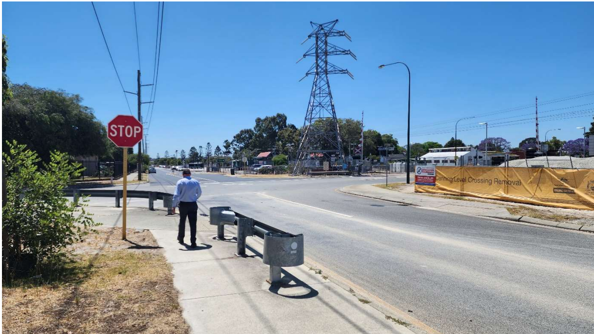
Photo 14: W-beam is too short to be effective and has non-crashworthy end treatments.
