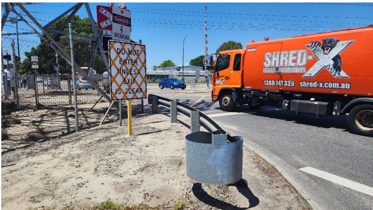
Photo 13: W-beam is too short to be effective and has non-crashworthy end treatments.
