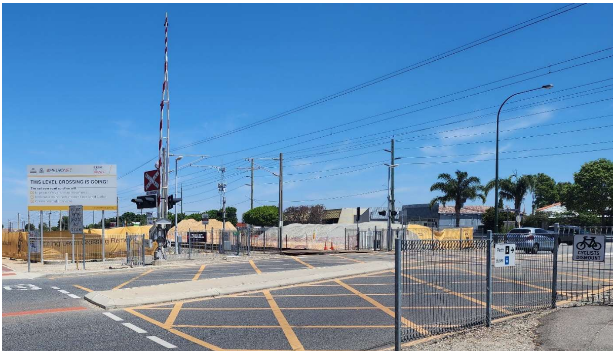
Photo 5: The level crossing is scheduled for removal as part of the upcoming Metronet projects.
